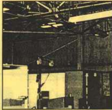
Conventional unit heaters replaced on this loading dock and in six other areas had a payback period of less than two years.
