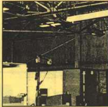
Conventional unit heaters replaced on this loading dock and in six other areas had a payback period of less than two years.
