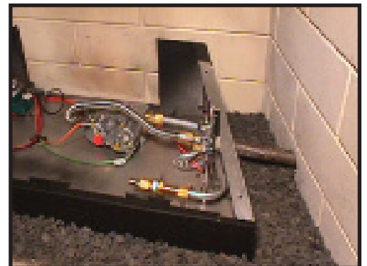
Figure 5 - Gas Line Connection
